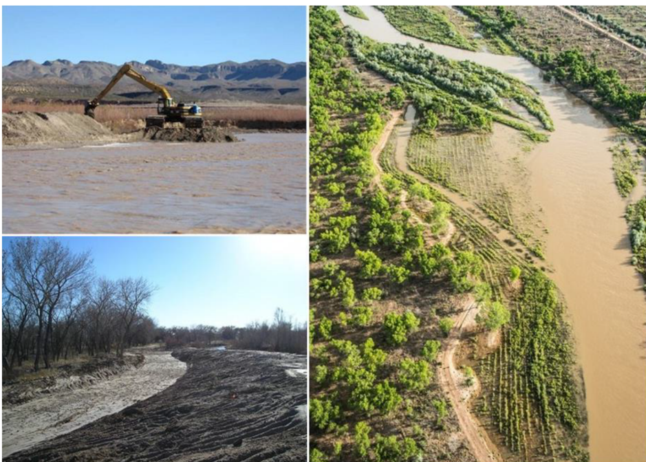
FIGURE 3 Amphibious caterpillar excavating a floodplain (upper left, SWCA), a terraced bankline (lower left, SWCA) and the Corrales floodplain site (right, Todd Caplan), all on the Middle Rio Grande, NM
