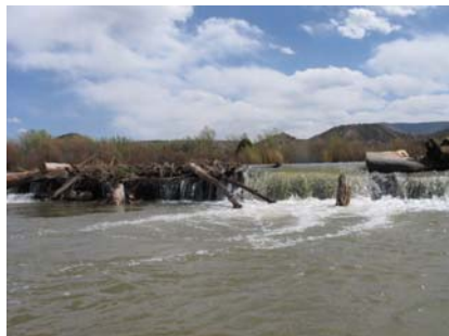
Most irrigation diversion dams along the reach are constructed mostly from pieces of concrete and woody debris. Photo: April 2008.
