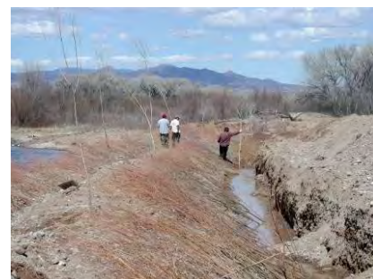
Willow installation at a swale constructed at Cochiti Pueblo. (Photo Credit: Parametrix)
