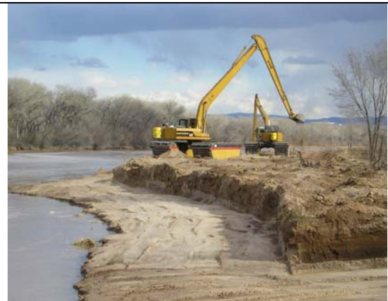
Figure 3.6.1.2. Bankline cut and embayment construction at a site in the I-40 to Central subreach. (Photo provided by Anders Lundahl, Interstate Stream Commission)
