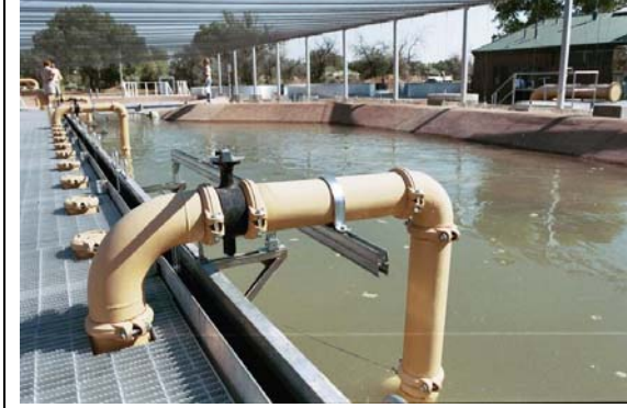
Figure 3.4.1.1. Filtration system in the Albuquerque BioPark Rearing and Breeding Facility.
