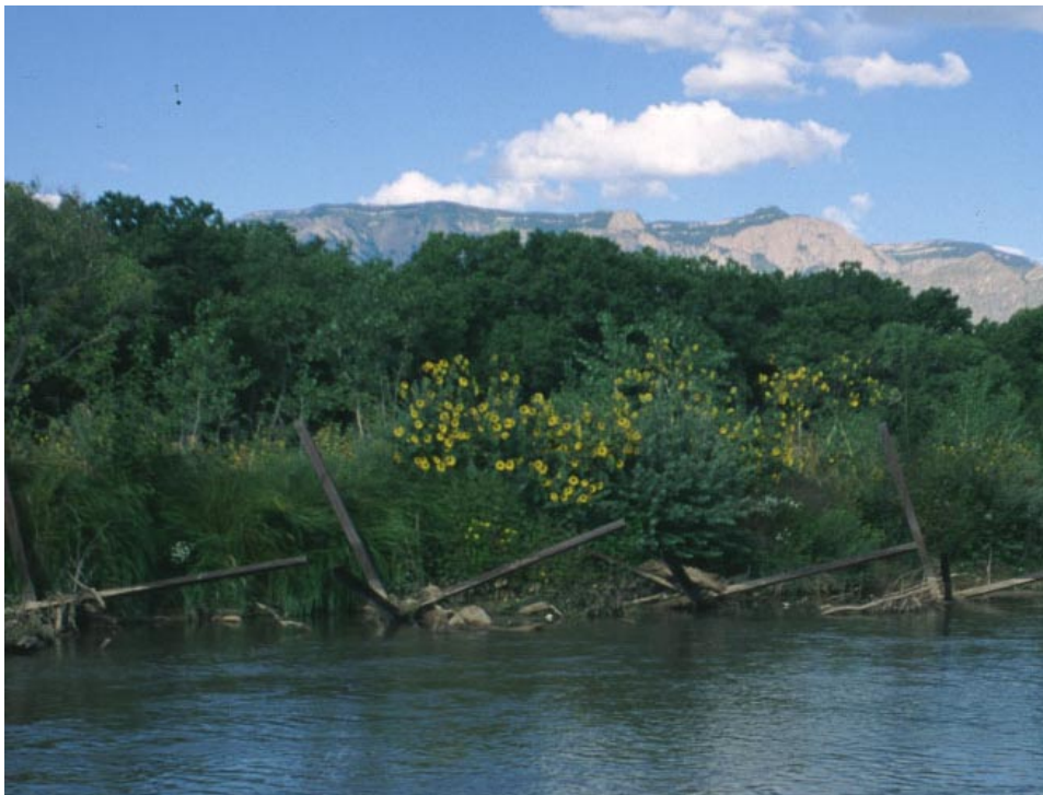
Figure 3. Photo of Kellner Jetty Jacks along the eastern bank of the Rio Grande. Banks have remained stable since jetty jack installation during the late 1940s to early 1950s
