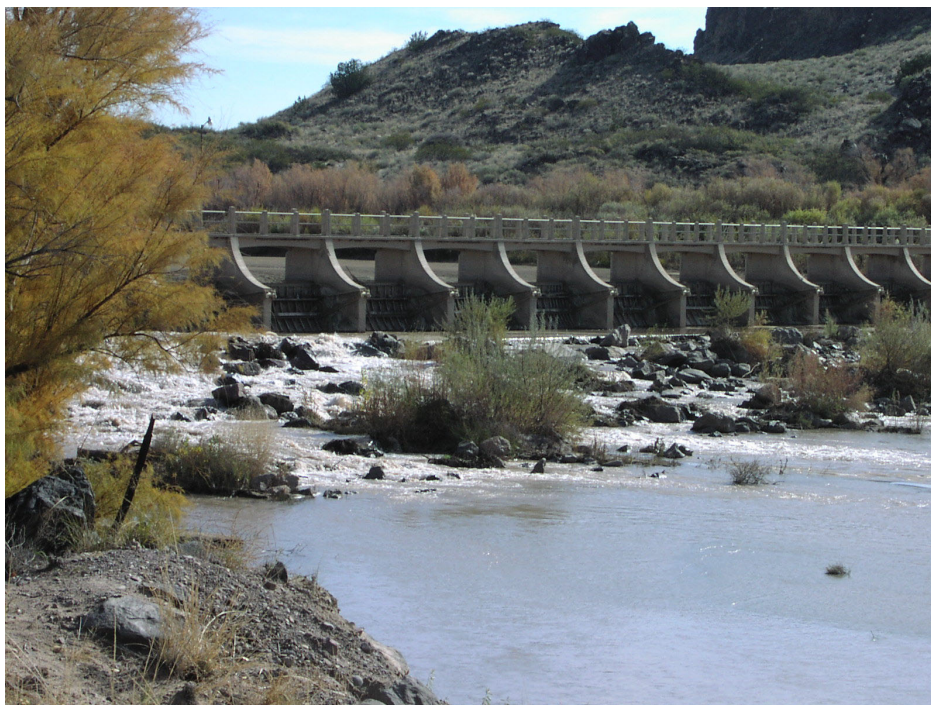
Figure 2. San Acacia diversion weir, viewed from a downstream perspective, is currently a barrier to upstream fish passage. (photo by D. Cowley, Nov. 23, 2002)
