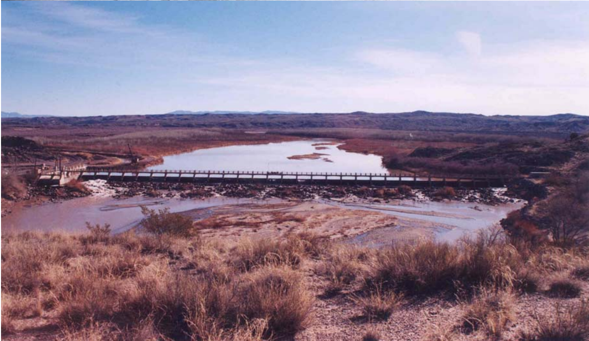
Figure 3. San Acacia Diversion Dam in 1952 (upper photo) and 2002 (lower photo). In 1952, gates are nearly buried in sediment. By 2002, there has been over ten feet of degradation downstream from the dam.
